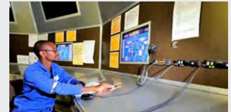
ERGO PLANT ELECTRONIC MONITORING SYSTEM
